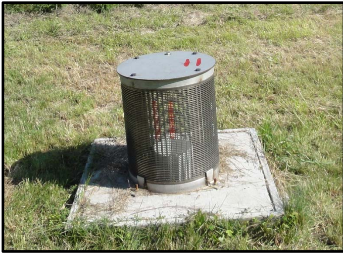
New seepage relief wells (shown above) will have a slotted, metal well guard and a reinforced concrete pad.
