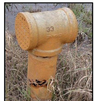
Existing wells to be replaced are T-shaped pipes that emerge from the ground along the length of the levee.
